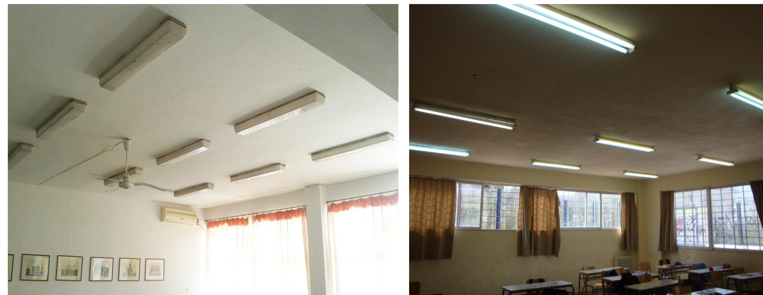
Figure 2. Typical artificial lighting system in classrooms of public domain school buildings. Left: T8 2 x 36W with electromagnetic ballast and milky cover (frosted diffuser). Right: T8 2 x 36W with electromagnetic ballast and without any cover (batten luminaire type)
